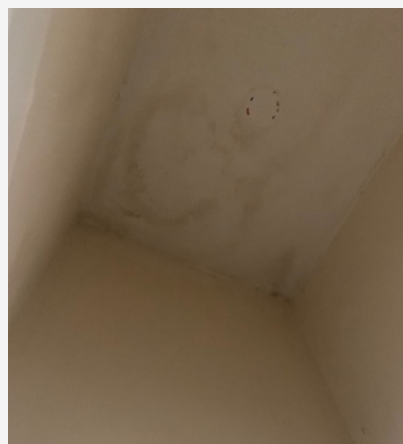
Damp on ceiling
